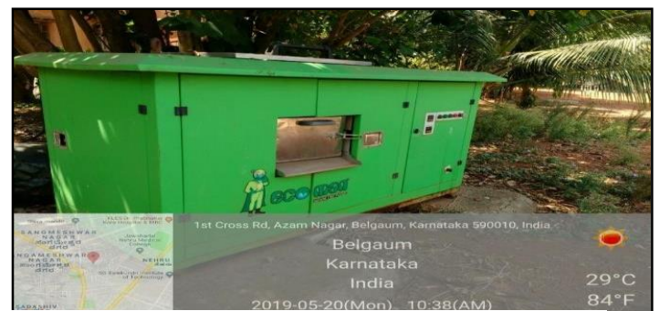
Waste recycling system
