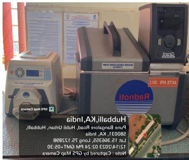
HEATER CIRCULATING PUMP
